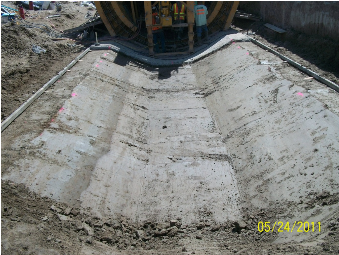
Subgrade prepared and trimmed to final shape just prior to placing the protective coating for a segment on the Weber Coulee North heading.
