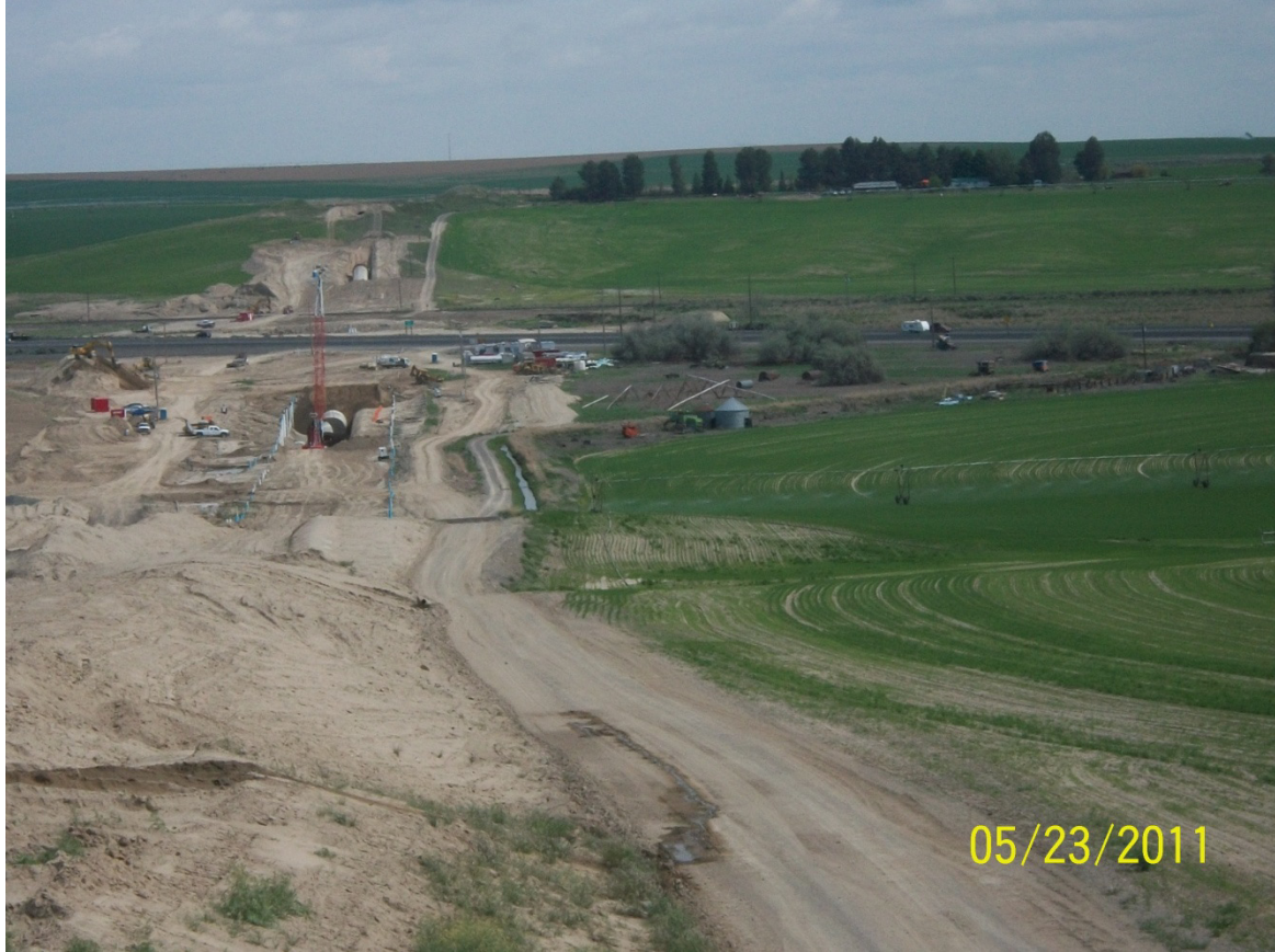
View from the south outlet structure of the Weber Coulee Siphon. Pipeline construction has proceeded quite some distance from the frontage roads where headings began. Siphon pipe construction now over 50% complete.
